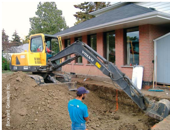
Above: The final contract should state that the pool will be built on the agreed upon location, using the agreed upon access route.
